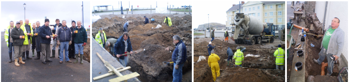
The first major step forward was the concrete pour for the foundations, then the weather held us up again!
